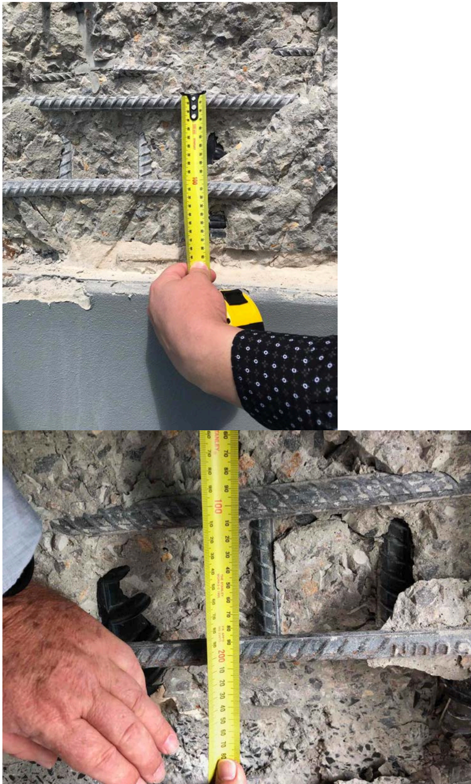
Figure 8. Photographs of the outside (top) and inside (bottom) of panel A at Level 10 just above hob beam adjacent to column 21, indicating N20 reinforcing bars at 100 mm centres in the lower portion of the precast panel. Note the exposed grout between panel A and the hob beam and the black plastic sheath for the joining dowel (top photo, right of tape measure).
