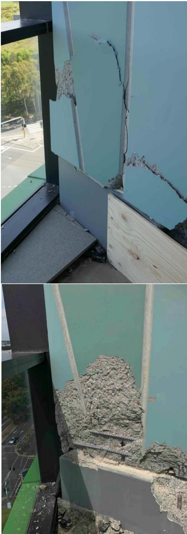
Figure 5. Damaged precast Panel A at Level 10 above column C21, before (top) and after (bottom) broken section of concrete removed.
