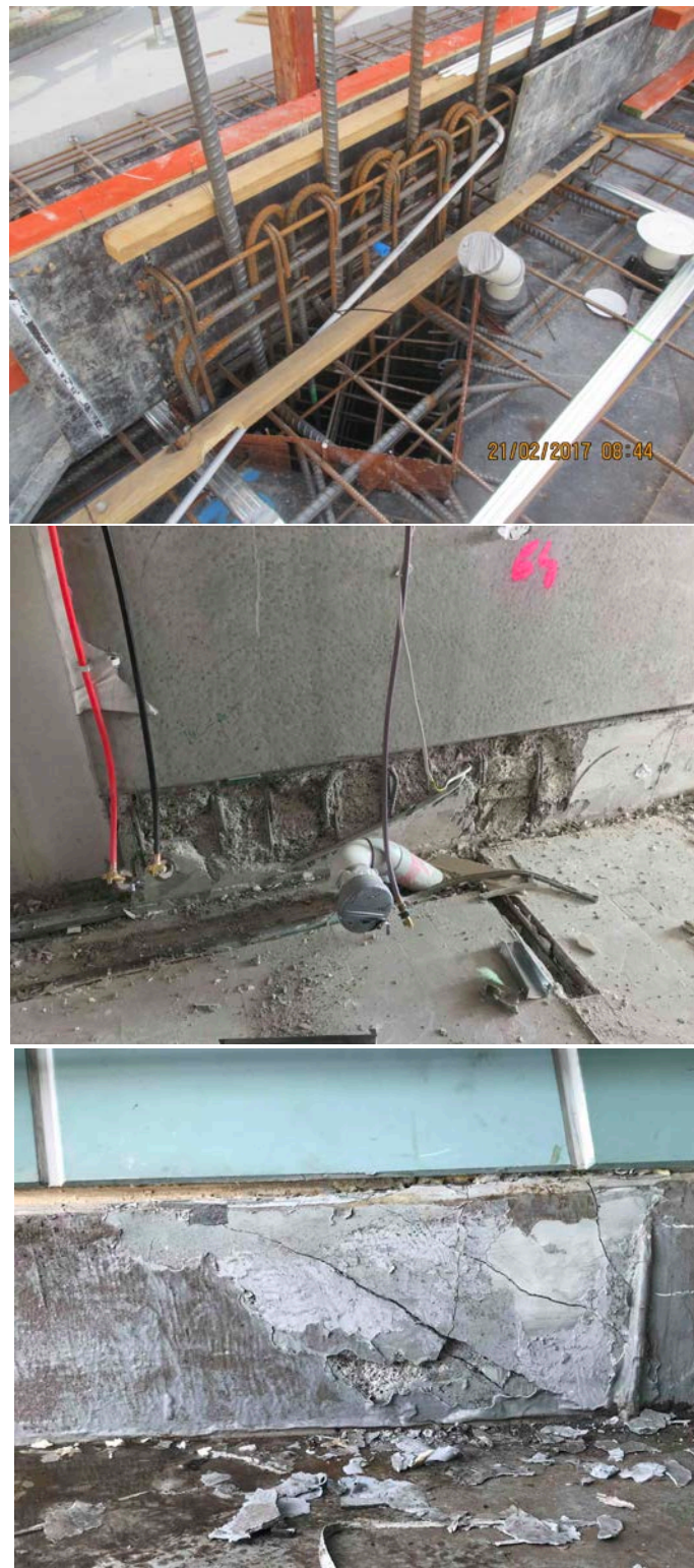
Figure 7. Photographs of the hob beam in the vicinity of column 38 at level 10, prior to pouring concrete (top photo), inside the building on 8 January 2019 after cracked concrete cover removed (middle), and outside on 8 January 2019 after the garden and waterproof covering removed (bottom). Note the positioning of the reinforcing bars, the encroachment of the column bars into the cover zone, the lack of anchorage of some horizontal bars, and the encroachment of a conduit into the concrete cover zone. The vertical dowel bars that engage with the precast concrete panels can also be seen in the top photograph.
