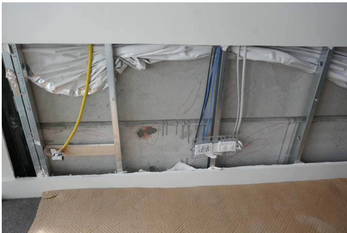
Figure 11. Photograph of the hob beam and panel on Level 4 near column C2 with red lines indicating minor cracking.
