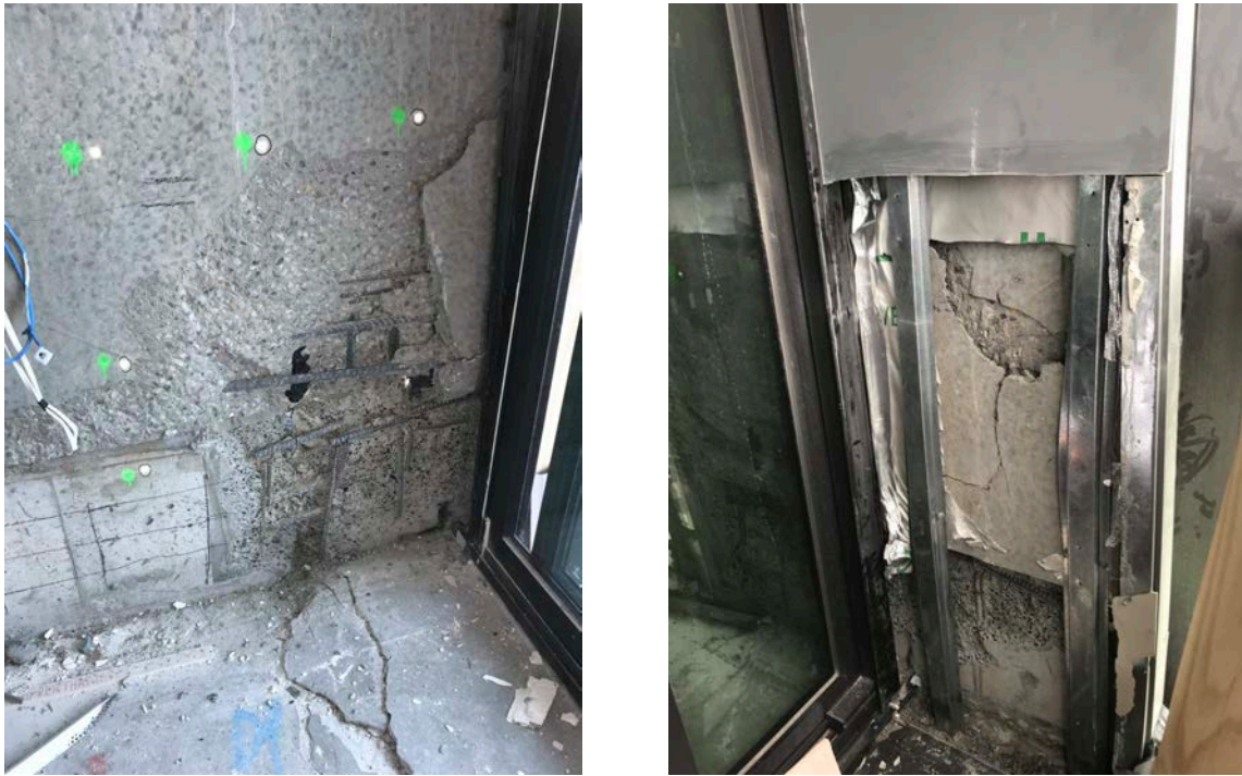
Figure 20. Hob-beam and precast wall panel at Level 10 in the vicinity of column C21 (apartment side) showing splitting of the precast panel and the damaged hob beam.
