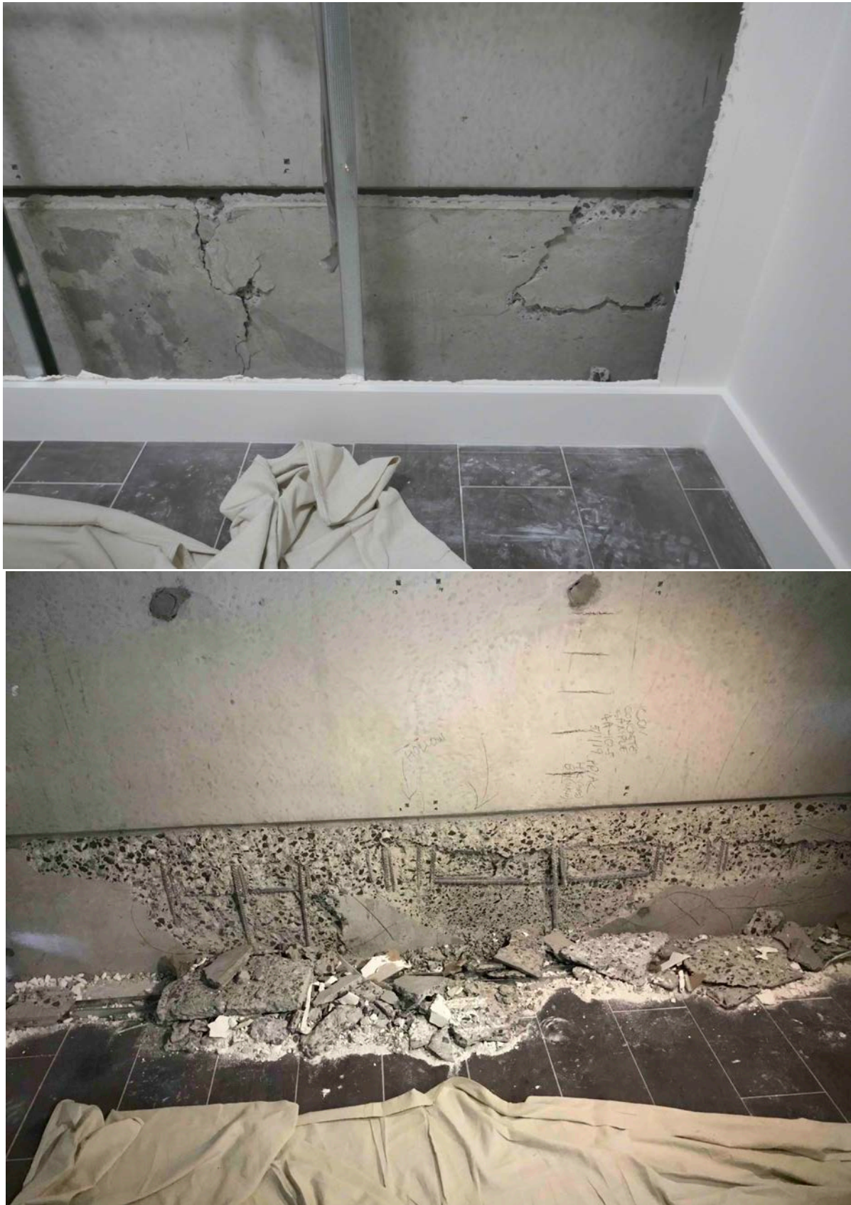
Figure 10. Photographs of the damaged hob beam on Level 4 near column C34 before (top) and after (bottom) cracked concrete removed.
