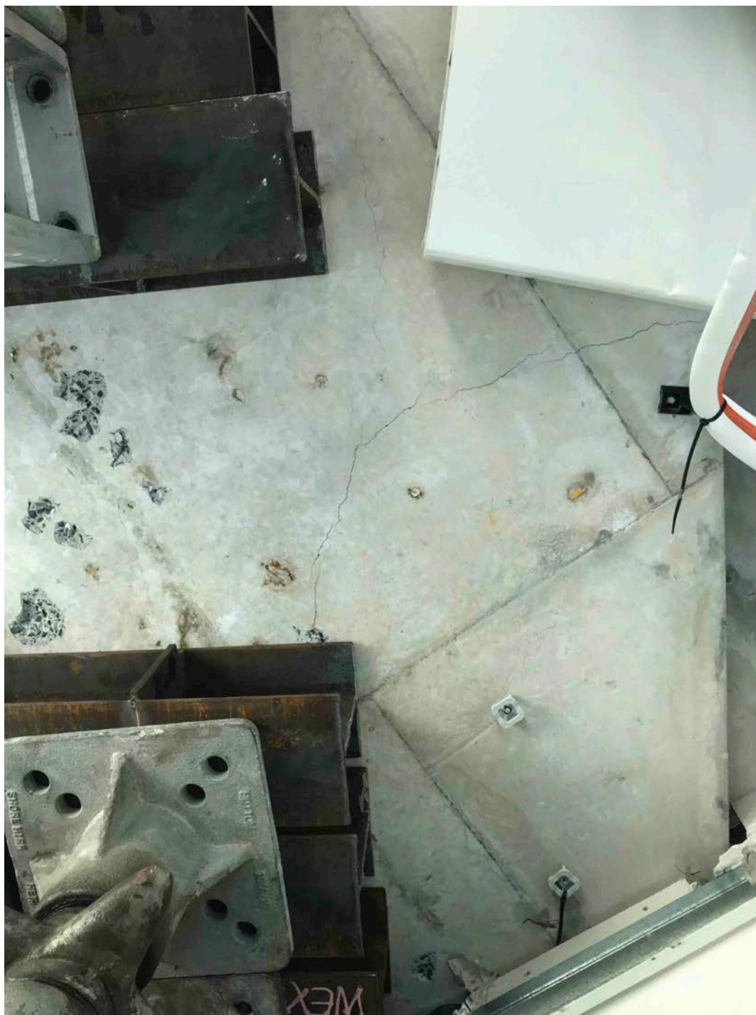
Figure 12. Photograph of a crack in the floor plate between Levels 3 and 4.
