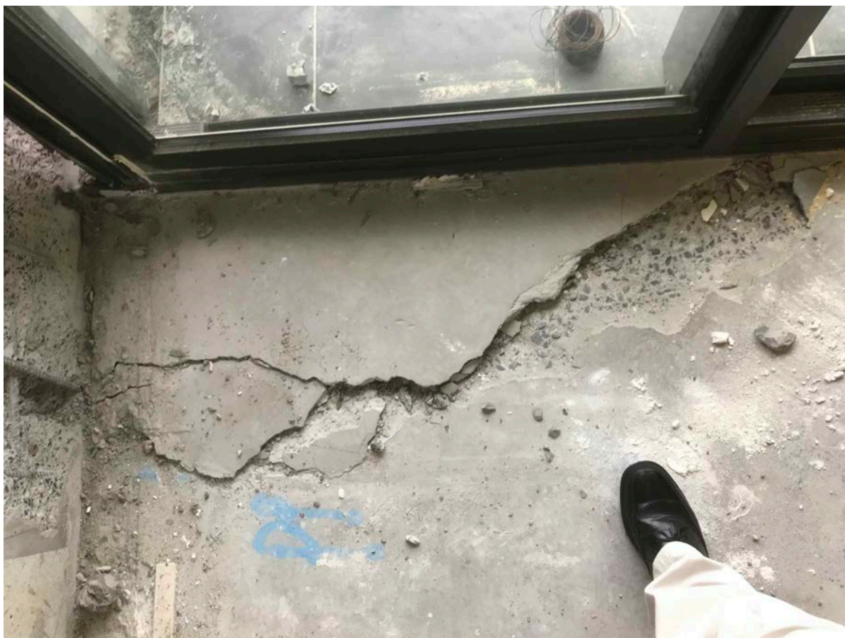
Figure 9. Photographs of the damaged floor slab adjacent to column C21 on Level 10.
