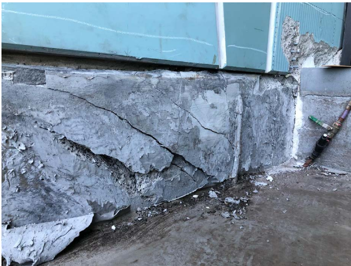
Figure 17. Hob beam at Level 10 in the vicinity of column C34 (outside) showing splitting along shear compression crack band lines.
