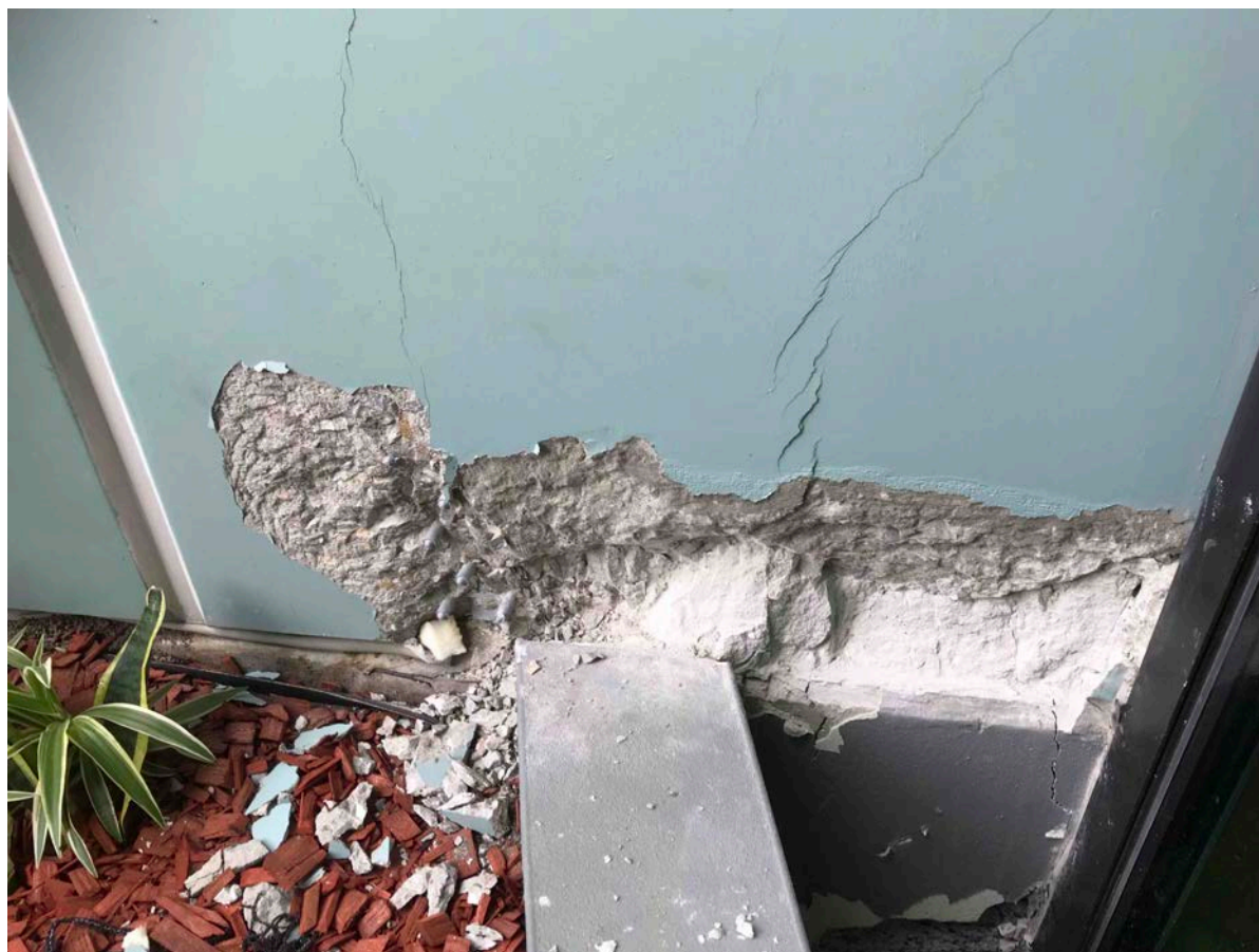
Figure 6. Damaged precast Panel A at Level 10 above column C38, after some broken sections of concrete removed.
